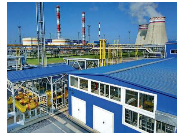
PHOTO 12. Gas treatment unit will provide fuel for the power generating units of Pregolskaya TPP in Kaliningrad
