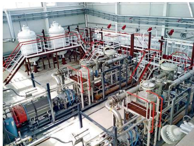
PHOTO 10. Compressor units feed associated gas to the South-Nyuryskaya GTPP
