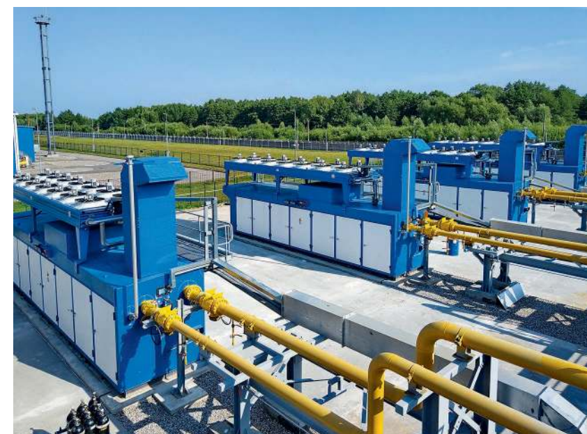
PHOTO 13. BCS consisting of four units is included in the comprehensive gas treatment system
