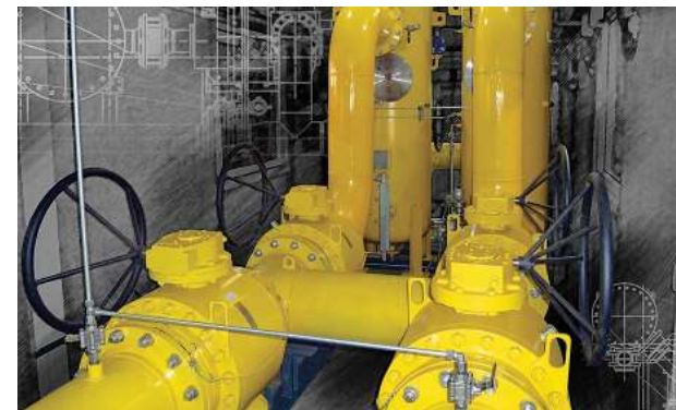
PHOTO 8. Process compartment of block-type gas treatment unit for the GTU-CHPP "Vostochnaya"
