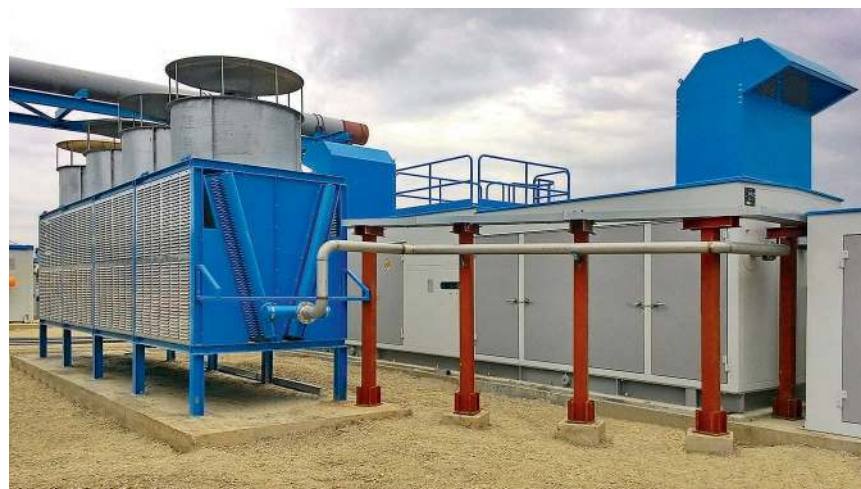
PHOTO 7. Block-module with process equipment and air cooler unit of CU
