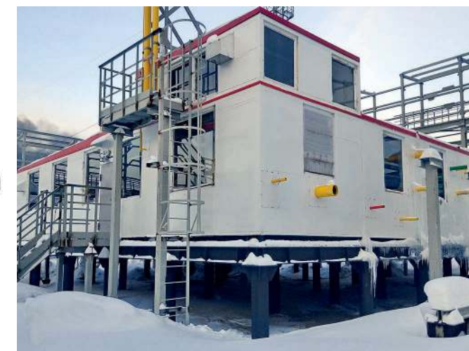
PHOTO 5. The FGTF-1 is installed at the CGCTP site of East-Urengoy licensed area
